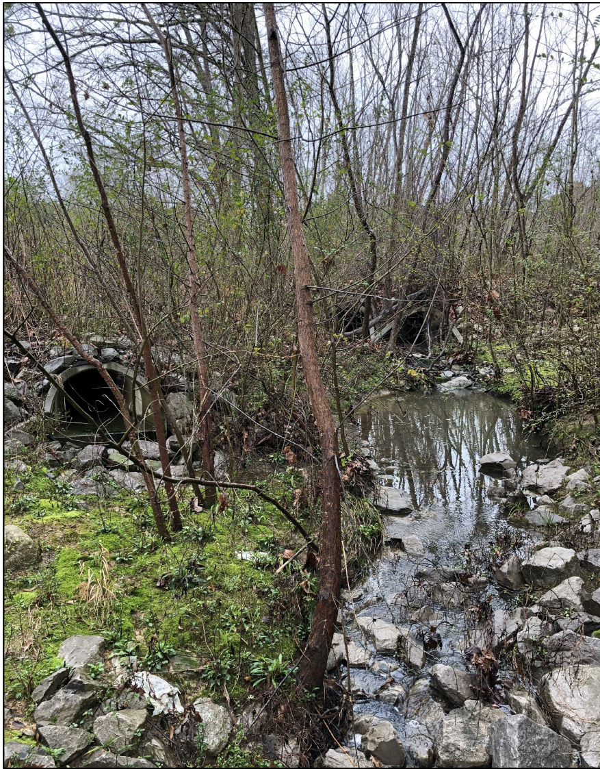
PHOTO 1: Ditch at Timber Ridge Detention Outfall
