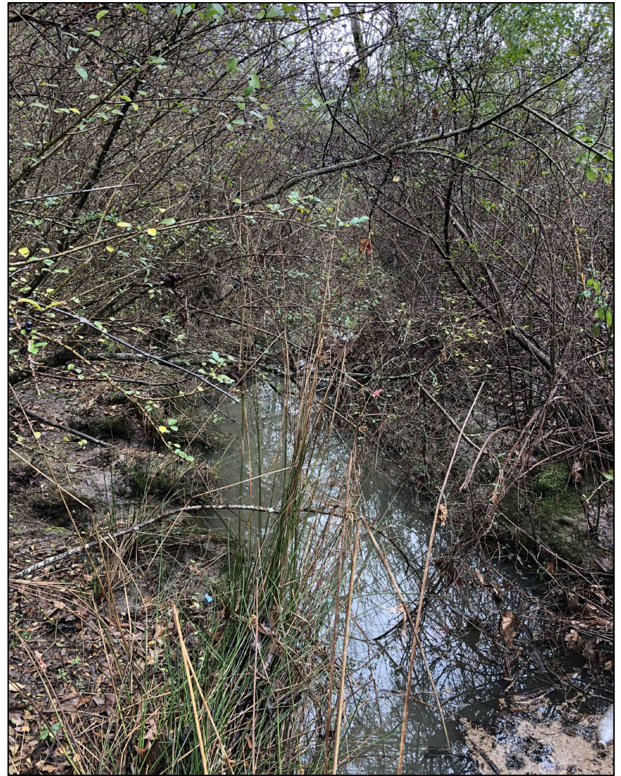
PHOTO 2: Ditch Downstream of Timber Ridge Detention Outfall
